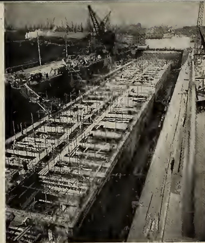
2. The parts of the "Mulberry" harbors were all built in Britain. The job kept 20,000 British workers working at top speed; 865,000 tons of reinforced concrete had to be cast in six months. Above are shown some caissons under construction in British yards.
